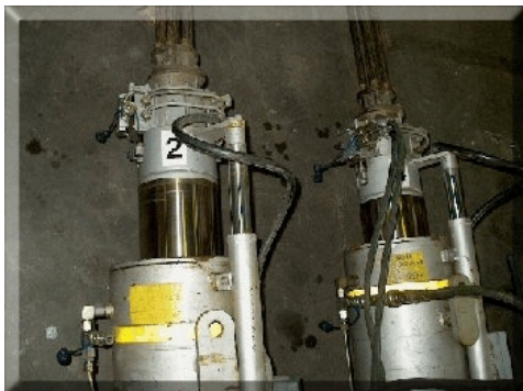
Picture 2: Lunac 2+ pistons after 7 years being exposed to various tough offshore conditions do not show any observable wear or corrosion.
